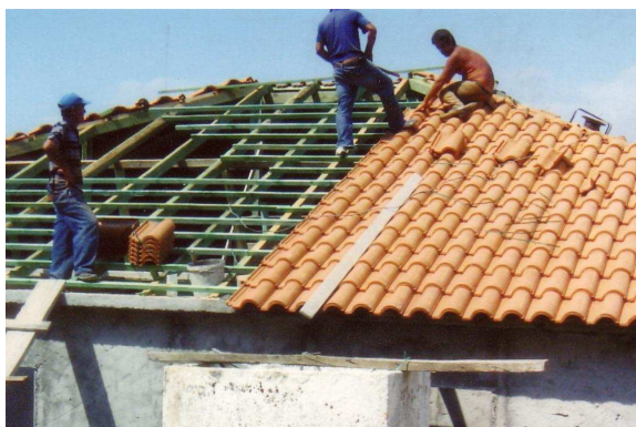
The reconstruction of the roof was only one of many building jobs
